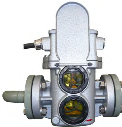
Fig. 19 Buchholz Relay on an arc suppression coil
