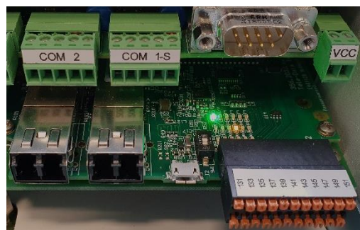
Fibre optical connection (2 x Ethernet-LC) at Level II; REG-DA Com ports at Level III
