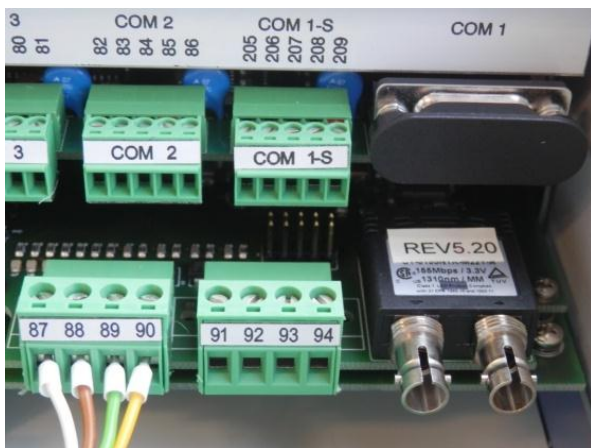
Fibre optical connection (1 x Ethernet-ST, XW93) at Level II; REG-DA Com ports at Level III
