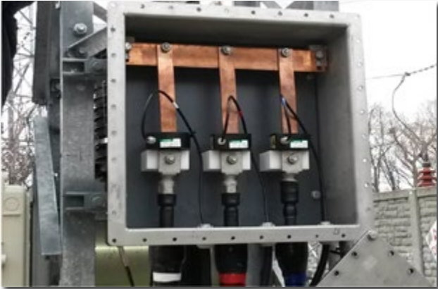
HFCT installation on OUTDOOR TERMINATIONS, inside grounding box.
